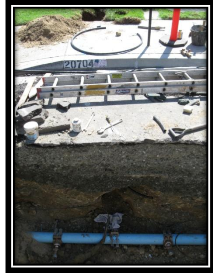
Service pipeline routed underground towards meter.
